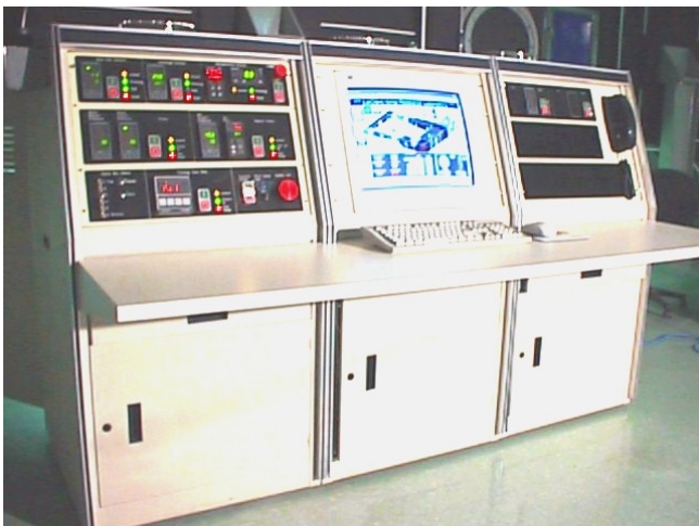
Figure 6: Master Control Console
